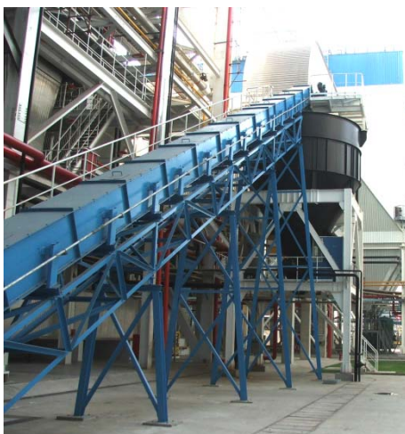
Figure 8: SSC Discharging to Dewatering Bins
