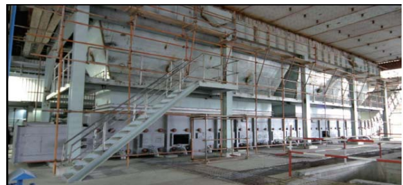
Figure 14: DRYCON Installed Under the Boiler Discharge
