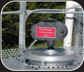
Measuring polystyrene in a polymer manufacturing facility.
